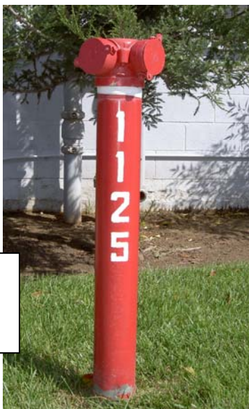
Fire Department Connection
