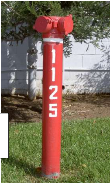
Fire Department Connection
